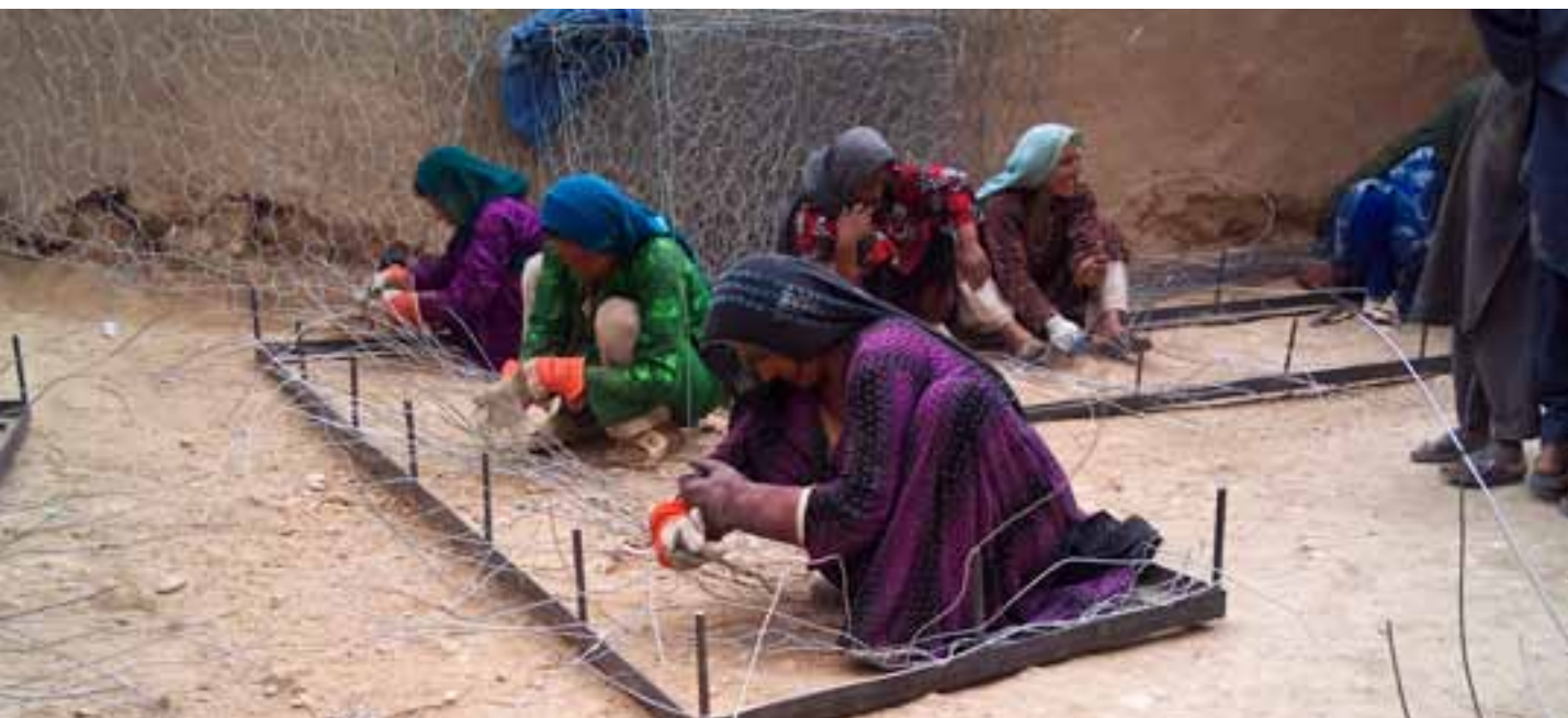
Women preparing wire baskets known as gabions as part of the Rural Access Improvement Project funded by Sweden in northern Afghanistan. The gabions will be filled with stone and used to rehabilitate roads in the Sar-e-pul and Samangan provinces. Photo: UNOPS
